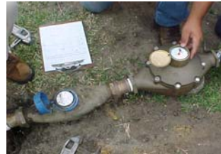
Old meter on left new meter on right
