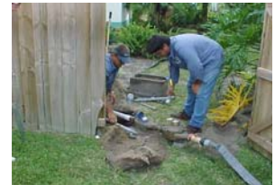
B. Klemm and E. Garay notice the flow and gallons measured on both meters.
