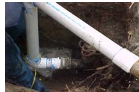
Pipes and fittings going to old meter (See Number 5).
